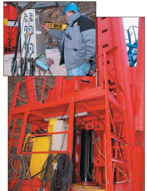
▼ Enerpac synchronous lifting system with PLC-control unit used to lift temporary support towers during bridge construction.
