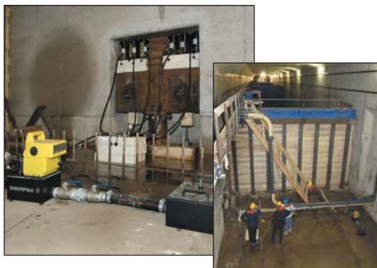
◀ Enerpac lightweight aluminum RAC-506 cylinders are ideal for wet environments such as this tunnel under the river (Holland High-Speed Train Line).
